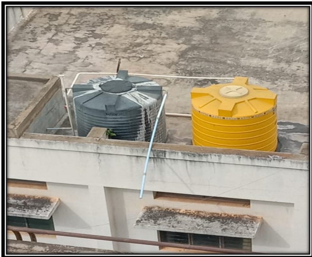
Photo: 9 Water Storage Tank
