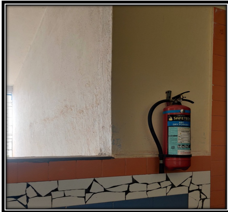
Photo: 14 Fire Extinguishers
